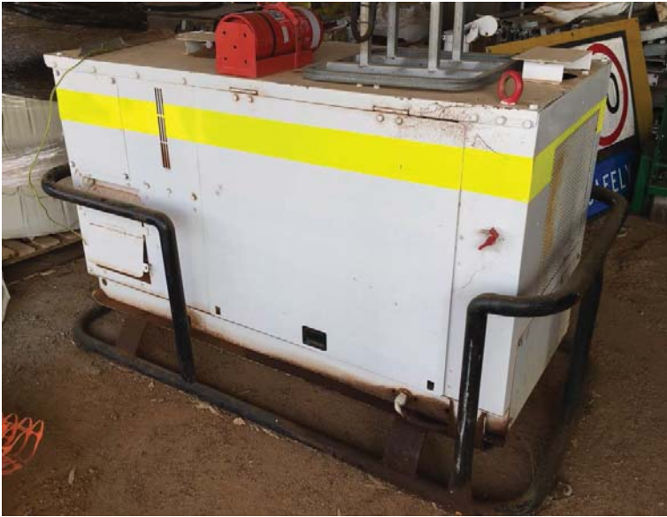
Above: Existing 23KVA Generator located at the Depot.
